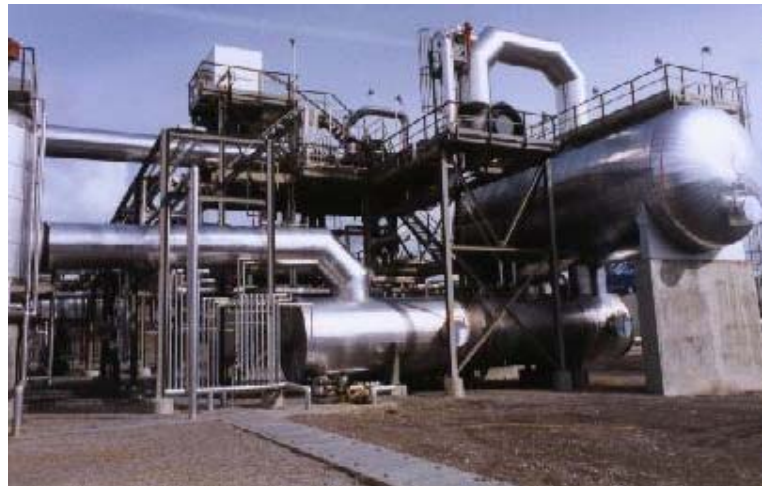
Claus® H 2 S oxidation plant
